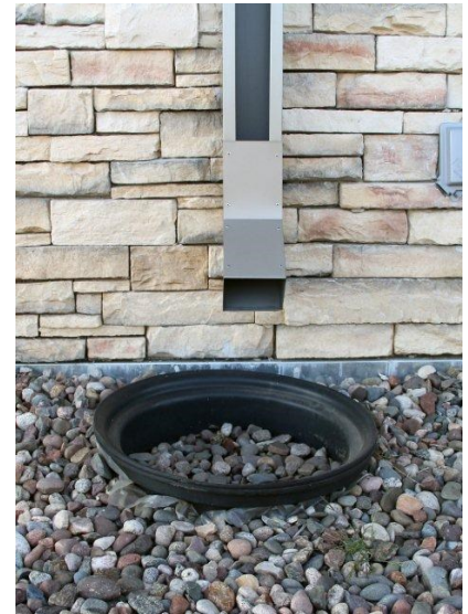
Rainwater is filtered by mesh and rocks before entering a collection tank.
